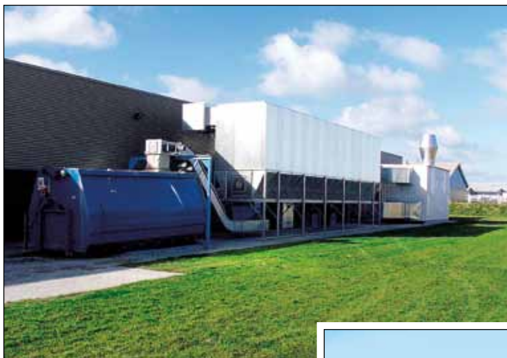
Aagaard chain filter at Danish furniture joinery with heat exchanger for return of air to the factory and with an Aagaard chip conveyor system for the transport of wood chips to a container.
